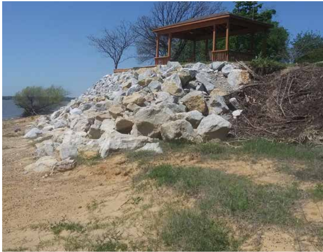
Figure 2. Rock blanket at Site 1; large (beige) rocks placed in 2020; smaller (grey) rocks added in 2024.
