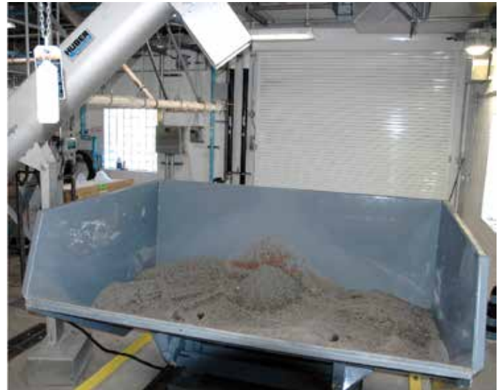
Phosphorus recovery dropping into a bin at a wastewater treatment plant that serves 2.2 million people. This phosphorus will be repurposed instead of sent down river.
