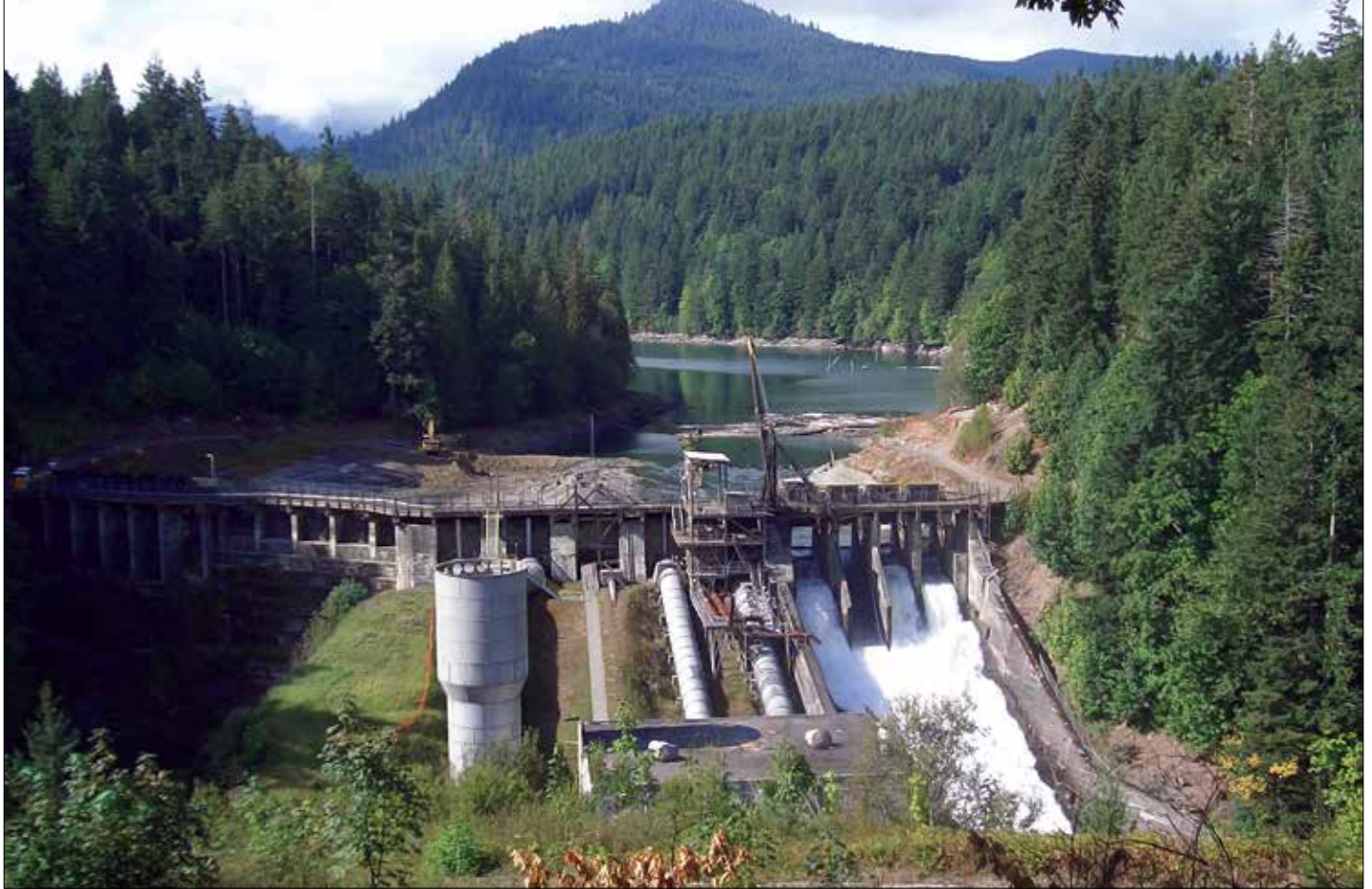
Figure 4. Elwha Dam early in the deconstruction process. Water has been diverted to the spillway on the right to lower the Lake Aldwell. Source: Creative Commons. Photo by Ben Cody.
