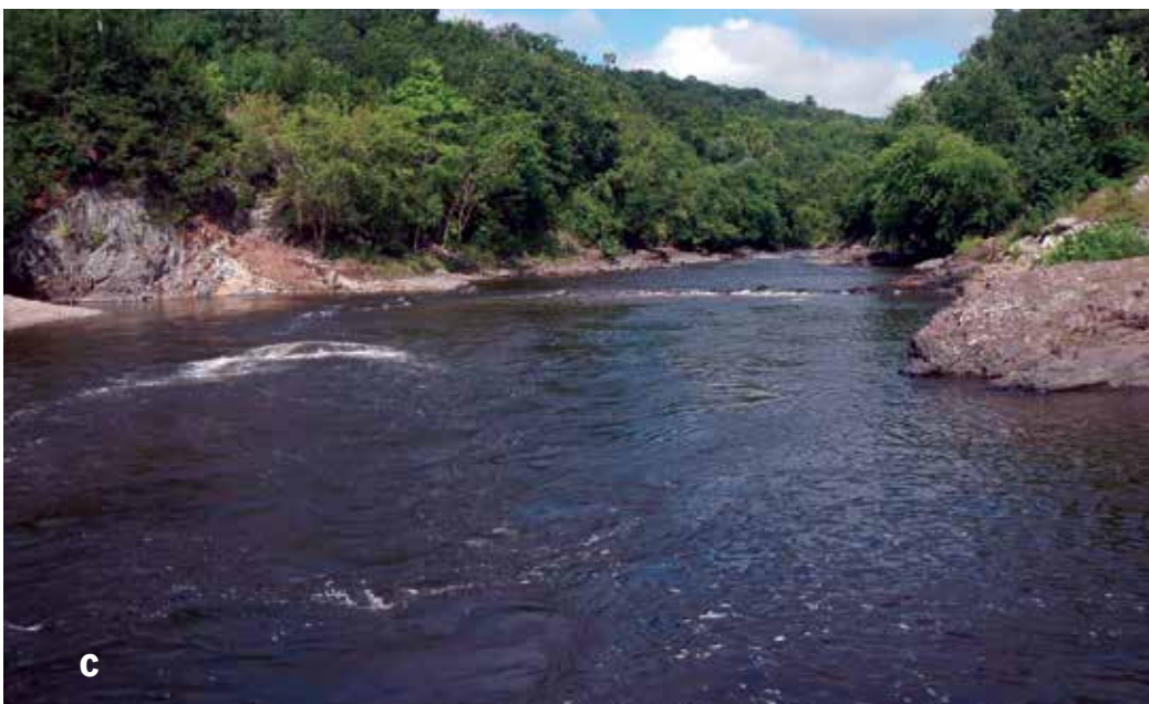
Figure 5. Spoonville Dam: (a) before removal, (b) during construction, and (c) after removal.
