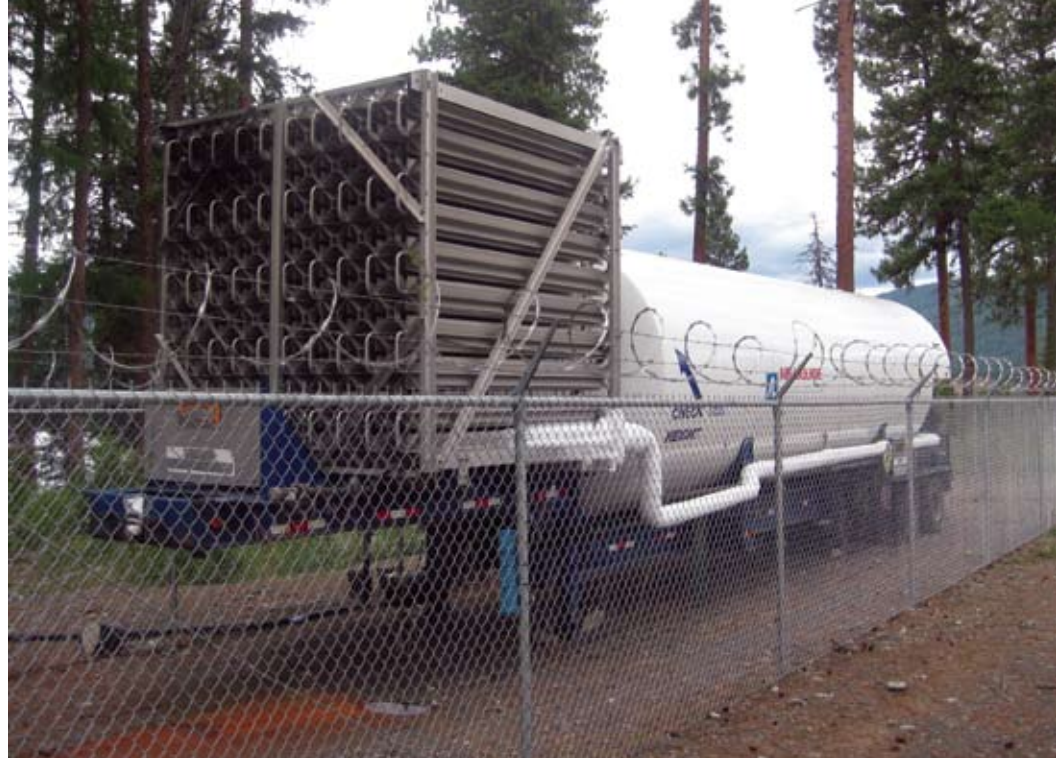
Figure 4. Liquid oxygen storage tank and evaporator on the shore of North Twin Lake. The storage tank can hold 6,000 gallons and the system can deliver 4,300 kg/day of gaseous oxygen to the lake.
