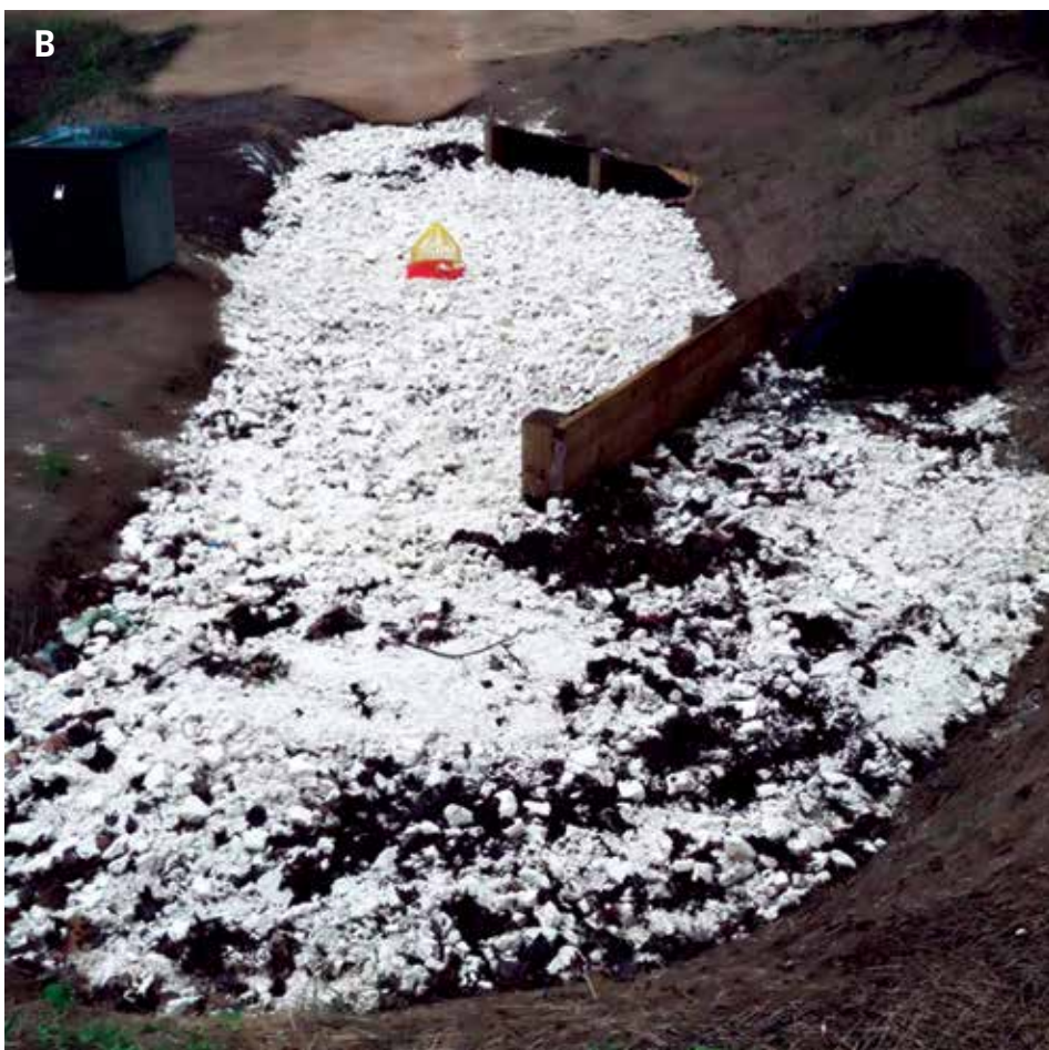
Figure 3. First-of-their-kind enhanced sand filter with 5 percent reused iron filings and spent lime filter (A) made of dried, drinking water treatment residual (B). Designed by Barr Engineering for the Ramsey-Washington Metro Watershed District in Minnesota. Photo A, Brian Huser; Photo B, Keith Pilgrim.
