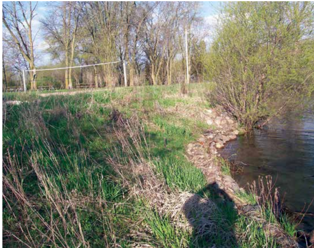
Figure 3. The public beach sand was moved up and away from the shore and glacial stone and native plantings were used to stabilize the shoreline.
