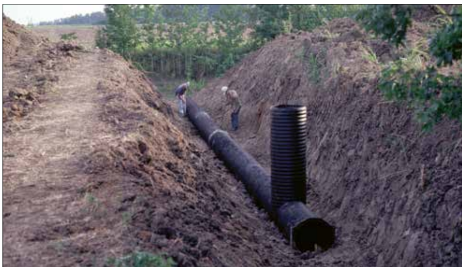
Figure 3. Grade Stabilization Structures, or “pipe drops” are an essential practice for eliminating gully erosion and head cuts along areas of high water flow and velocity, most often adjacent to near natural coulees or other water courses. NRCS file photo.
