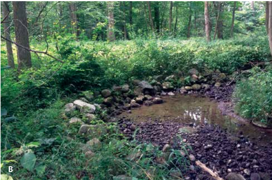
Figure 3. Putney Ditch streambank stabilization project during (A) and 8 years after implementation (B).
